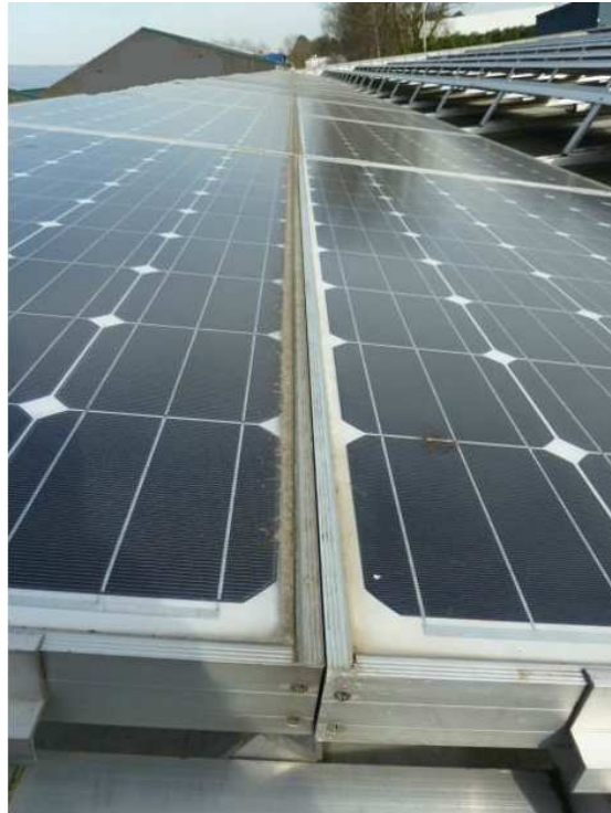
PV power plant (roof)
