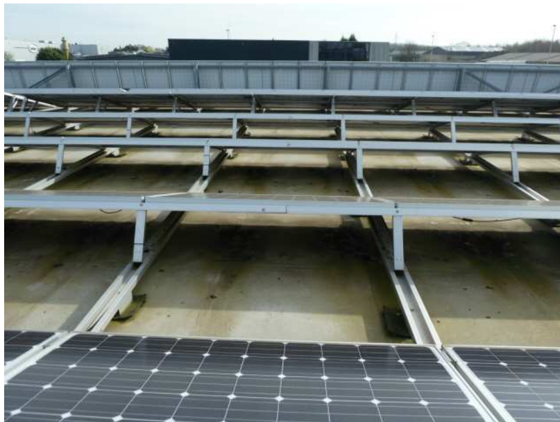
PV power plant (roof)
